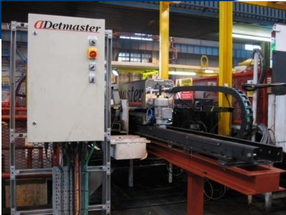
Picture 1 Detmaster 1300 MPH pinhole detection system installed on Shearing Line No. 5
