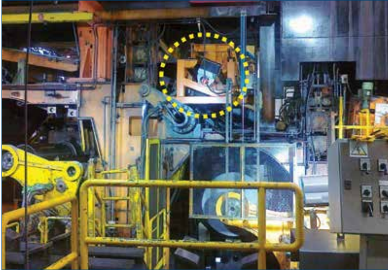
Roll mark detector integrated in the exit of a 5-stand tandem mill, inspecting all coils to the second coiler (on the left side).
